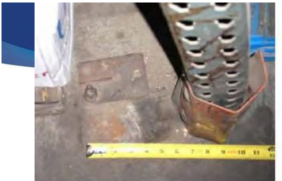
Damaged leg of storage racking needs to be repaired.
