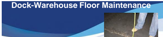
Pot holes create overturn and load drop hazards for lift trucks
